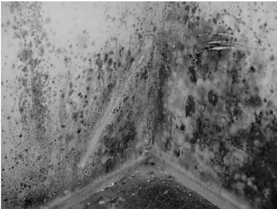
Example of mould inside a cupboard
